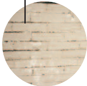
flaking or peeling paint
