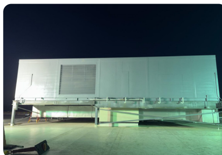
AHU Exterior After
