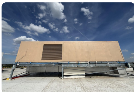
AHU Exterior Before
