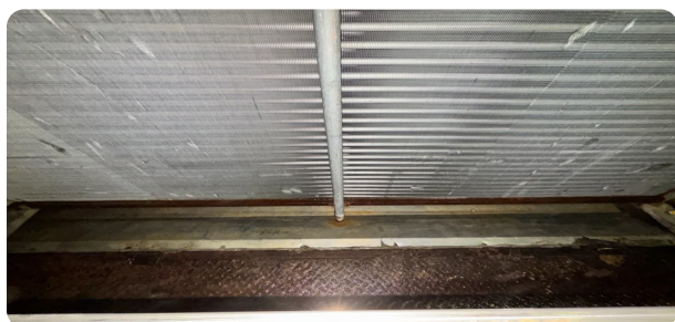
Before Drain Pan Protection
