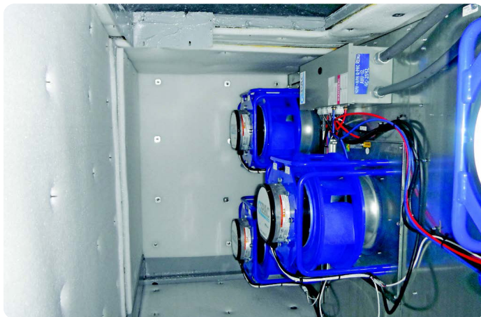
HVAC Insulation System
