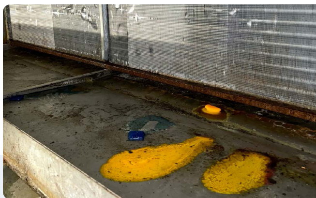
Drain Pan before
