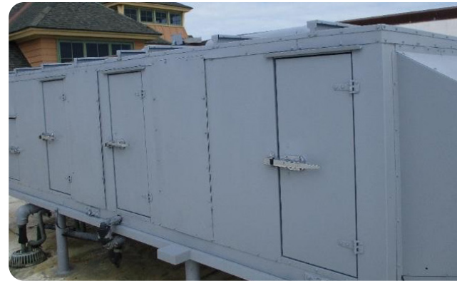
Air Handler Unit
